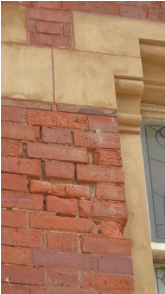
Late Victorian building repointed with cement mortar which has led to frost damage
