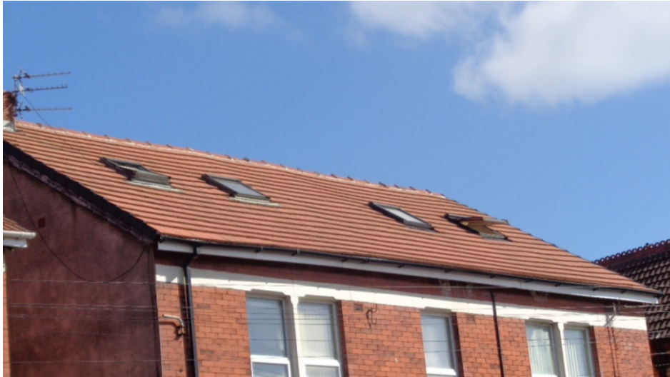
Roof lights which are higher than the front roof slope
